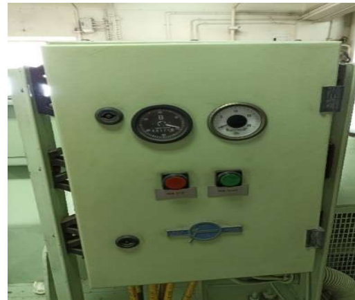
Gambar 8. Panel Start Emergency Generator
