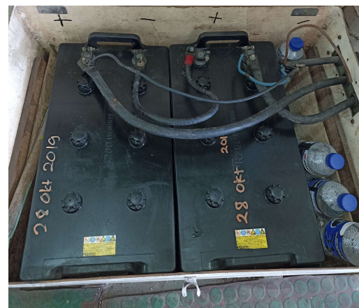
Gambar 15. Battery Emergency Generator
