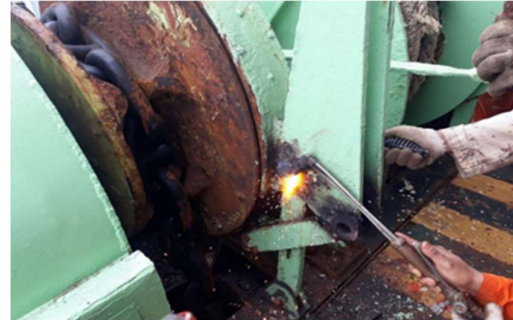
Figure 2. Corrosion of the Chain Link
