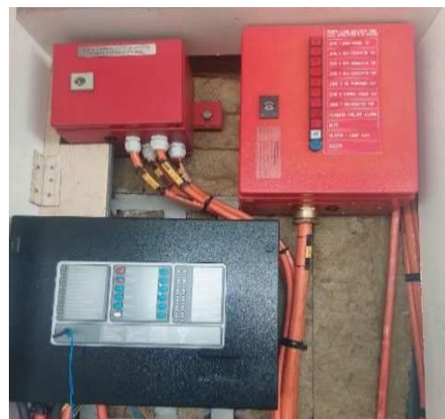
Gambar 3. Main Control Fire Alarm
