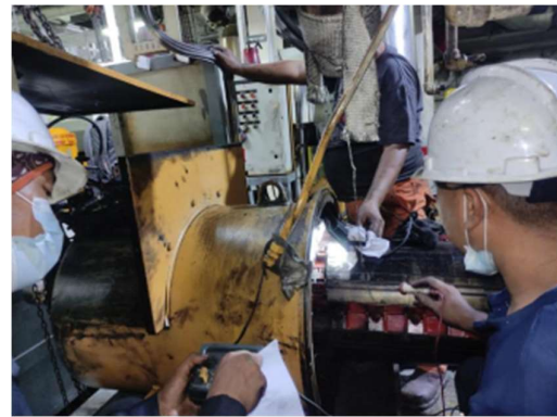
Gambar 6. Maintenance and Cleaning of Emergency Generator.
