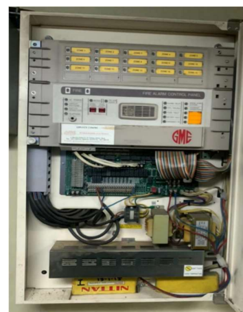
Gambar 1. Main Control Fire Alarm
